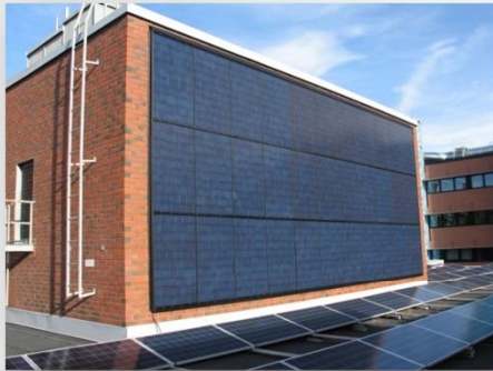
LUT PV PLANT (EXISTING)
